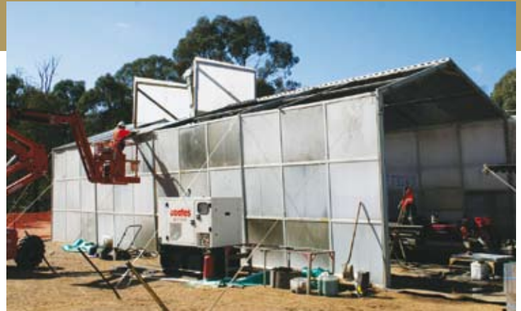
Above: The noise attenuation shed is erected to house the drill rig at New Moon.
