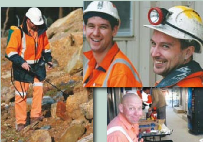
Above: Revegetation of the bund wall on Diamond Hill has progressed well over the winter. Environmental Officer Paul Ennor takes advantage of the winter sun to spray the weeds.
